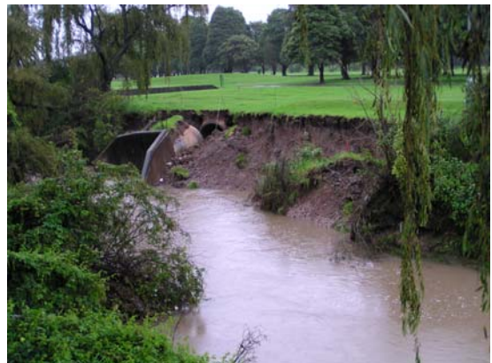
Bank instability and erosion, Freshwater Park, May 2003
