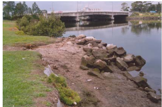
Bank erosion, Kendrick Park
