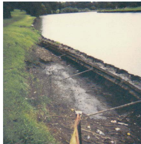
Collapsing sheet piling on Cooks River upstream of Riverview Road
